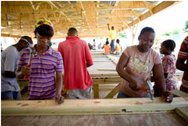
Guerdy Charles, left and Jenne Venson right, temporary CRS workers, construct a section of a transitional shelter at a prefabrication yard, Haiti, 2010, Photo Credit: CRS
