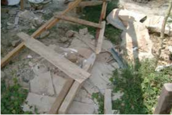
Construction materials are unsafely scattered over construction site Photo Credit: CRS
