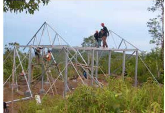
Construction in progress of 45sqm permanent housing in mountain village of Nias Photo Credit: Ariel Sadural for CRS
