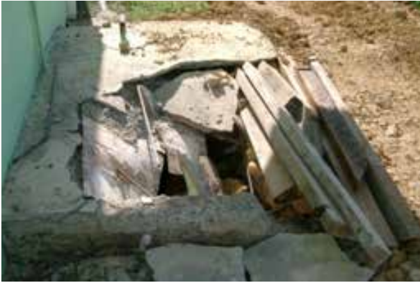
Site safety hazard Photo Credit: CRS
