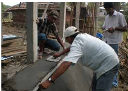
Plinth of flood-resistant shelter is being reinforced with chicken wire and concrete Photo Credit: Kirtimayi Mishra for CRS
