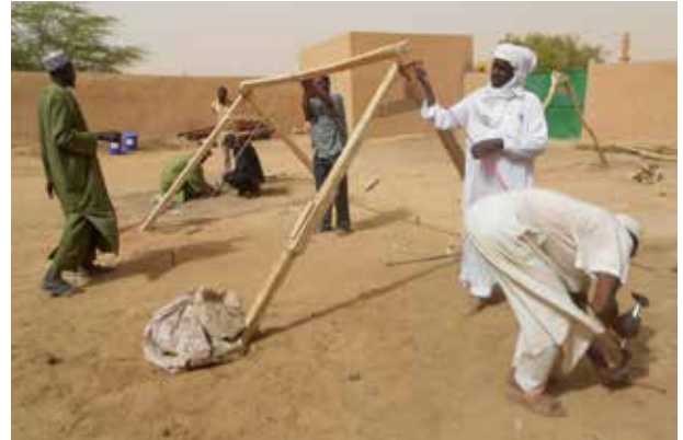
Construction training for host and affected communities and CRS staff of emergency shelter, Niger, 2012 Photo Credit: Seki Hirano for CRS
