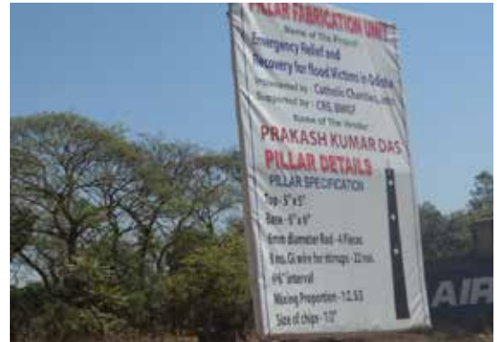
Reinforced concrete pillar prefabrication site for the structural frame of flood resistant shelter. Photo Credit: CRS
