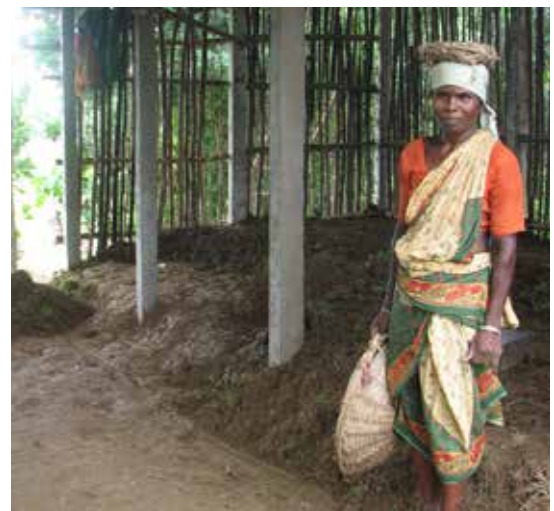
Owner creating the raised plinth around the concrete pillars. Photo Credit: CRS
