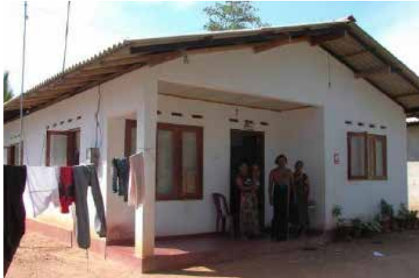
Pilot construction of transitional shelter in progress for post-tsunami shelter response, Sri Lanka Photo Credit: CRS
