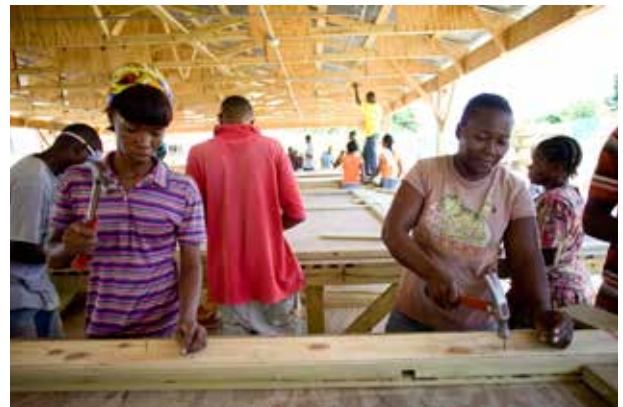
Prefabrication yard for T-shelters employed 50% women and 50% men. The manager reported that this created a balanced work environment and that women’s productivity was equal to others, Haiti earthquake response, 2010 Photo Credit: Benjamin Depp for CRS
