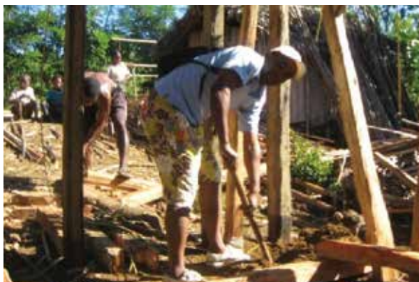
Pilot construction of shelter for training local community and craftsmen on cyclone resistant construction Photo Credit: Rumana Kabir for CRS
