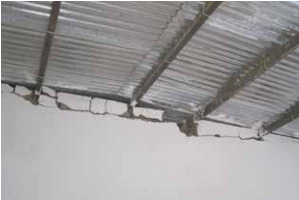
Sub-standard quality construction in a school made from stabilized earth blocks in Dafur, 2011 Photo Credit: CRS
