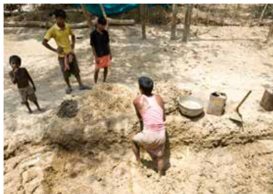
A neighbor helps CRS program participant Purna Chandra Dalai prepare a mud and straw mixture for his new home, built to be flood resistant using techniques and materials taught and provided by CRS. Photo by CRS
