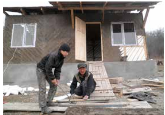
Winterized t-shelter with insulation layer under construction Photo Credit: Andrew Schaefer for CRS
